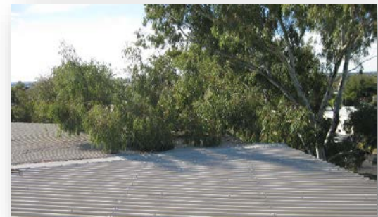
Overhanging trees deposit leaf debris and allow vermin to access roof areas
