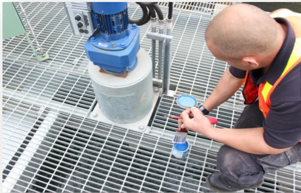
Paint being applied from an open can directly over a drinking water supply.
