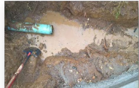
Poor pipe management - note ingress of soil and foreign matter into open pipe ends
