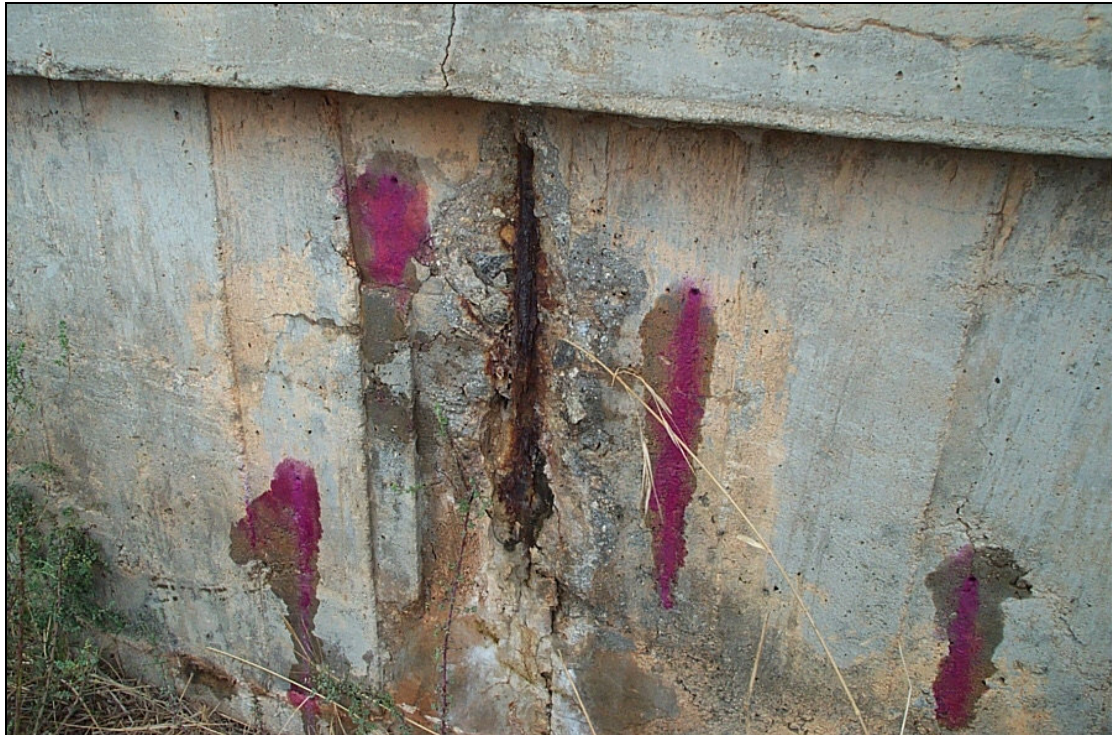
Figure 3 - purple tailings indicating that alkaline concrete has been detected
