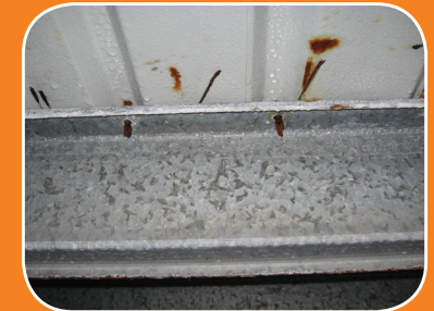
Corroded roof screws and safety mesh.
