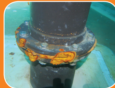
New ductile iron pipework corroding.
