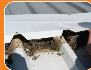
Ridge capping debris.
