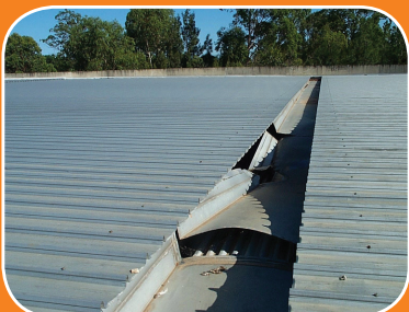
Box gutter collapsed.
