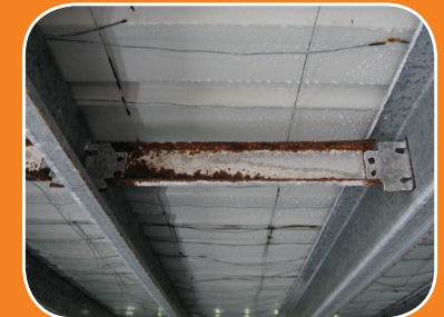
Corroded purlins and safety mesh.
