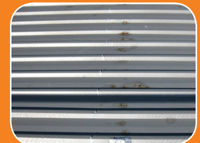
Roof sheet corrosion from safety mesh below.
