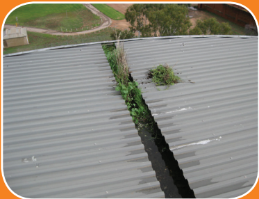
Box gutter blocked and overflowing.
