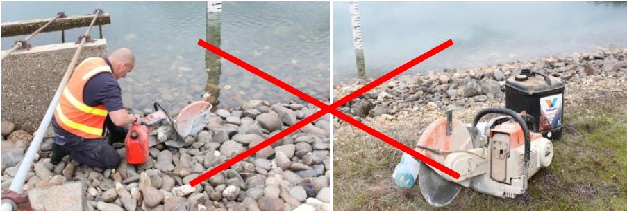
Filling up construction and maintenance equipment with petrol or oils directly next to a water storage without adequate spill control - note the lid left off the oil container
