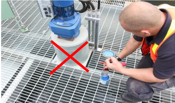
Paint being applied from an open can directly over a drinking water supply
