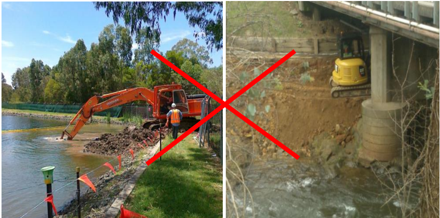
Excavation works can affect drinking water storages or catchments by stirring up sediment
