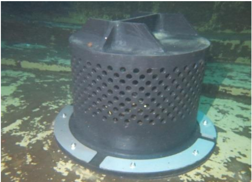
(Top) An outlet bell mouth level to the floor, scouring sediments into the downstream pipework. (Bottom) An HDPE safety screen with a sealed and raised base section solves the problem
