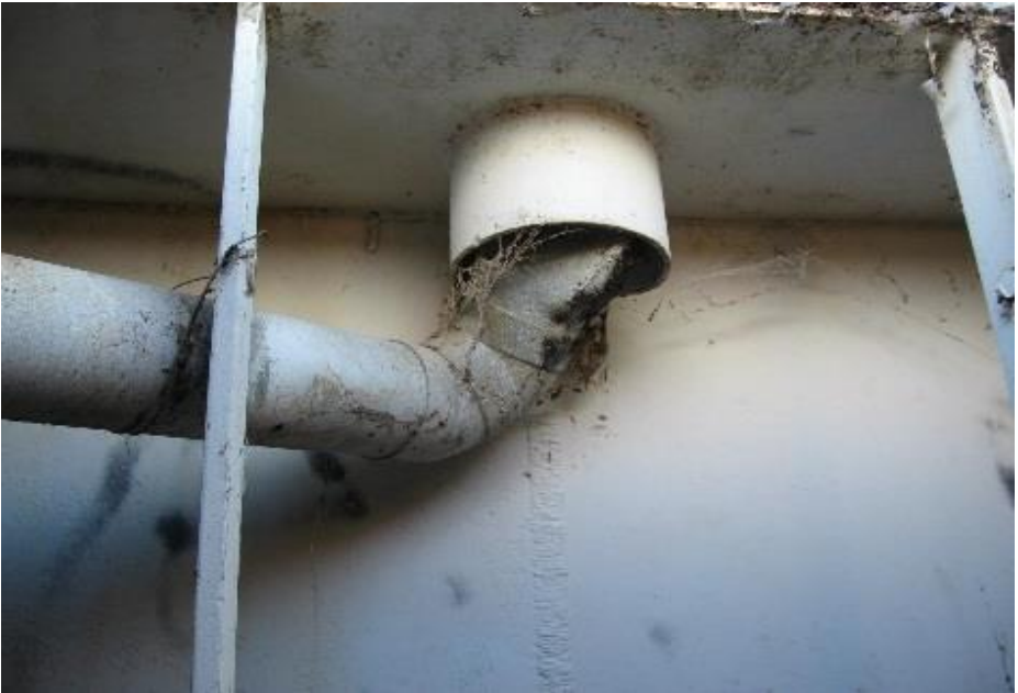
Roof drainage points not connected properly underneath, allowing storm water runoff and bird faecal material to enter the tank
