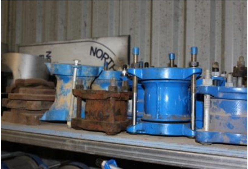
Mixed fittings (water and waste) which are accumulating dirt and contaminants
