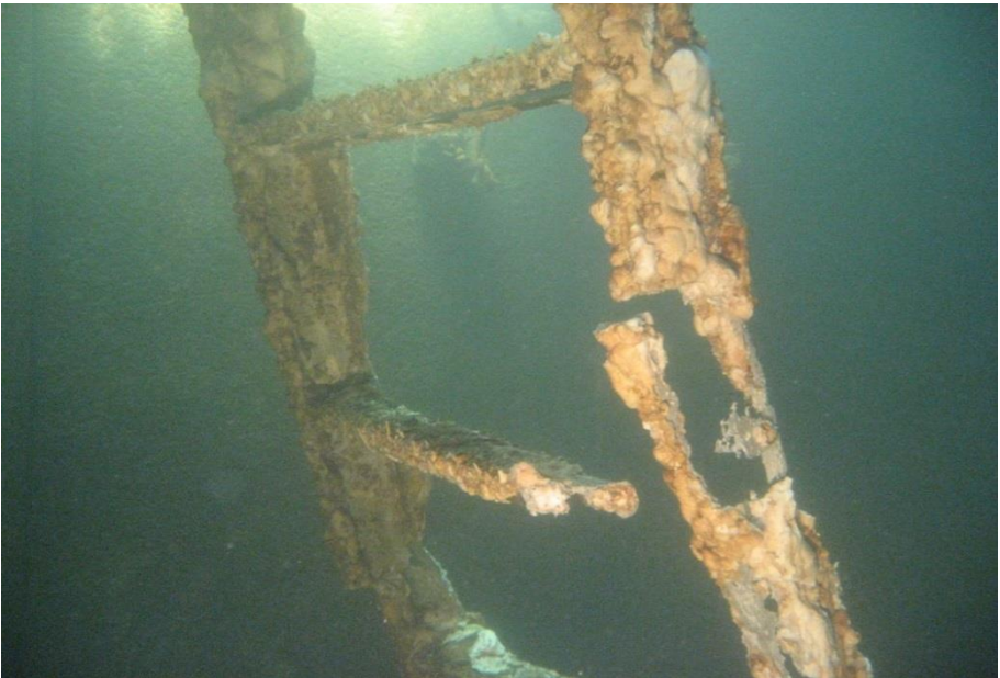
Corroded infrastructure will impact the disinfection residuals and should be replaced with more suitable materials
