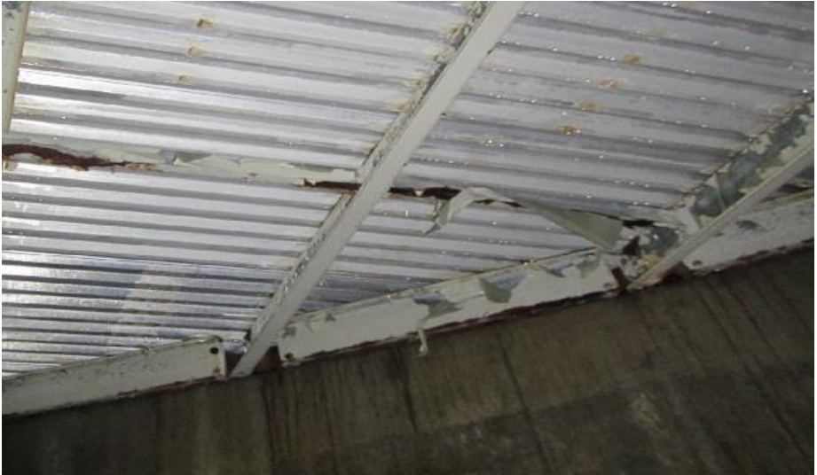
Protective coatings peeling off and entering the water due to the moist, chlorine environment
