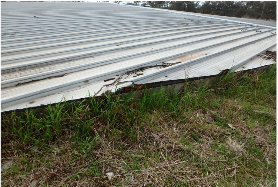
Gaps in storage tank roofs allow vermin and debris entry
