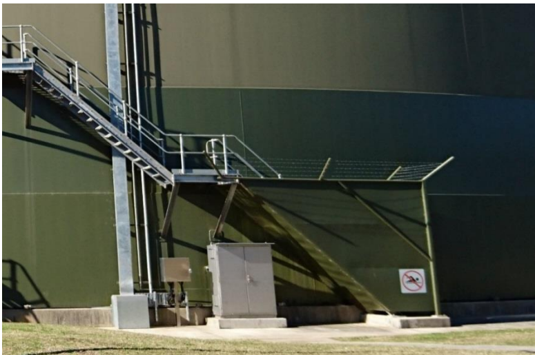
Poorly positioned fixtures and design allows for unauthorised entry to site
