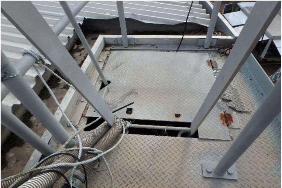
Hatch covers with gaps which allow bird, vermin or debris entry
