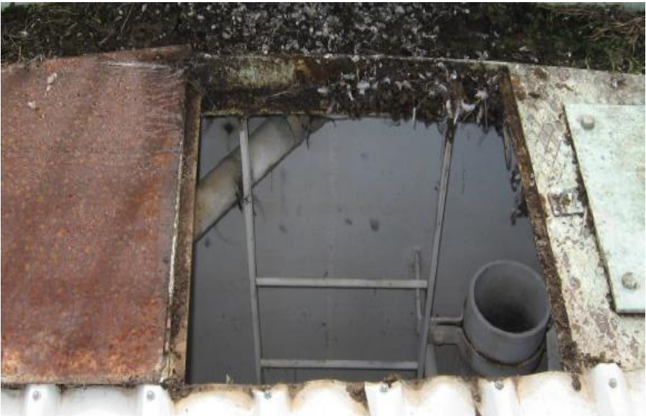
Hatches which are not raised or sealed allow bird faecal material to enter the tank
