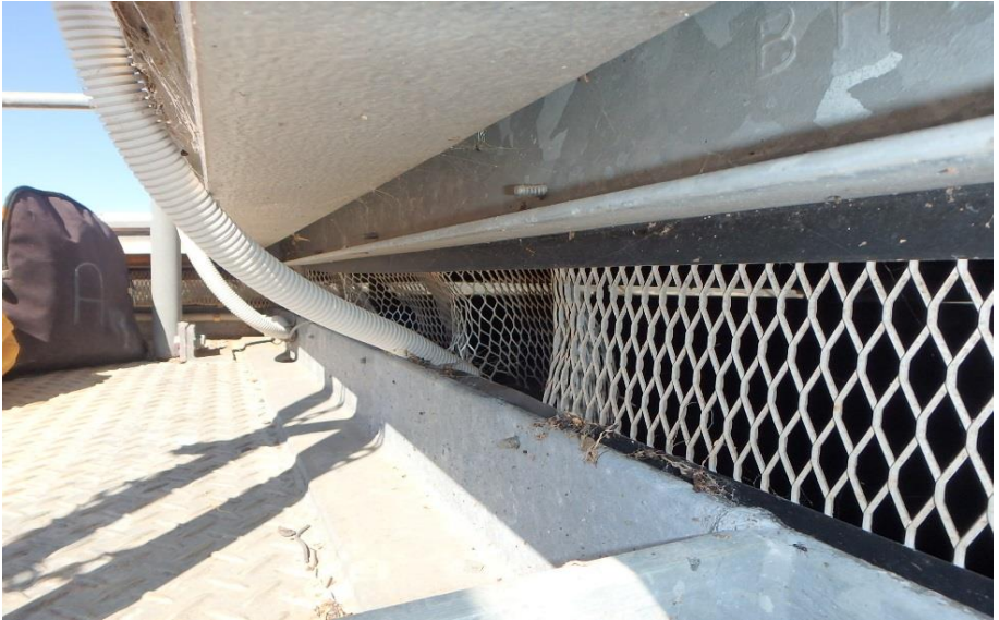
Electrical cable installation damaging vent mesh and creating vermin entry points
