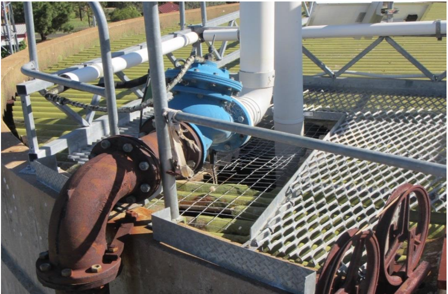
Features added to a tank without thought for protecting water quality. An unsealed hole in an asbestos roof after installing additional inlet pipework
