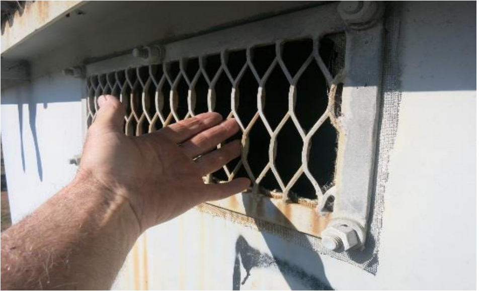
Large mesh holes allow dust, debris, insects, birds and vermin to enter
