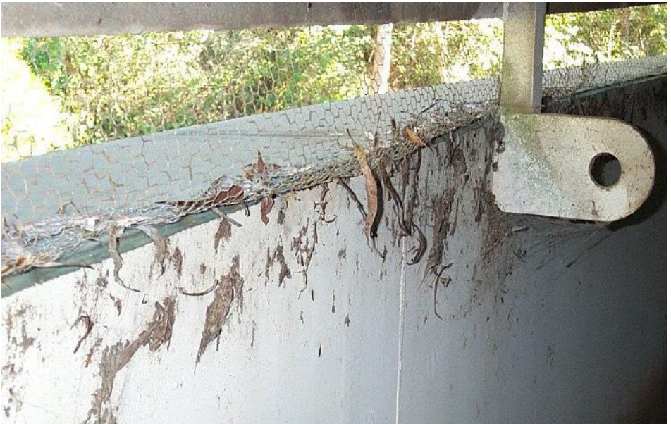
Accumulated leaf debris entering past the coarse vent mesh and subsequently falling into the tank
