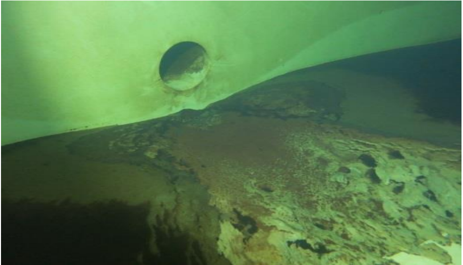
A wall mounted inlet and outlet penetration can disturb accumulated sediments during the filling and draining cycle
