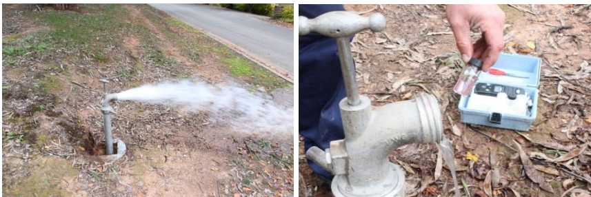
Mains flushing following a repair and a chlorine residual test being completed at nearest downstream hydrant to the repair
